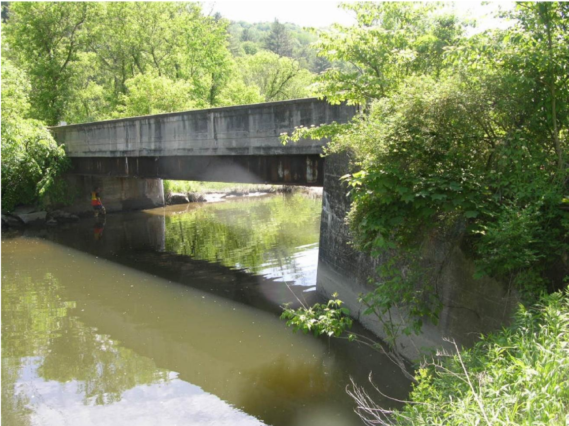
Looking downstream at waterway constriction
