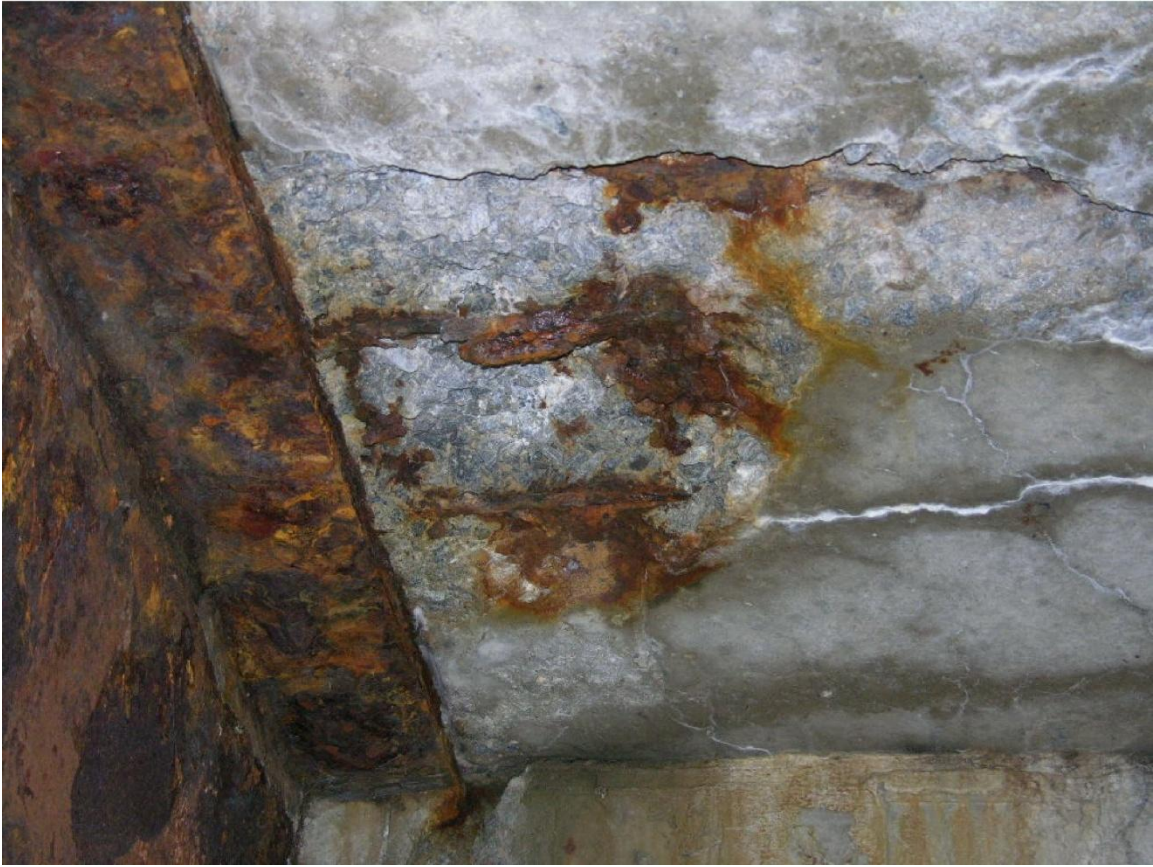
Deck and Girder Deterioration
