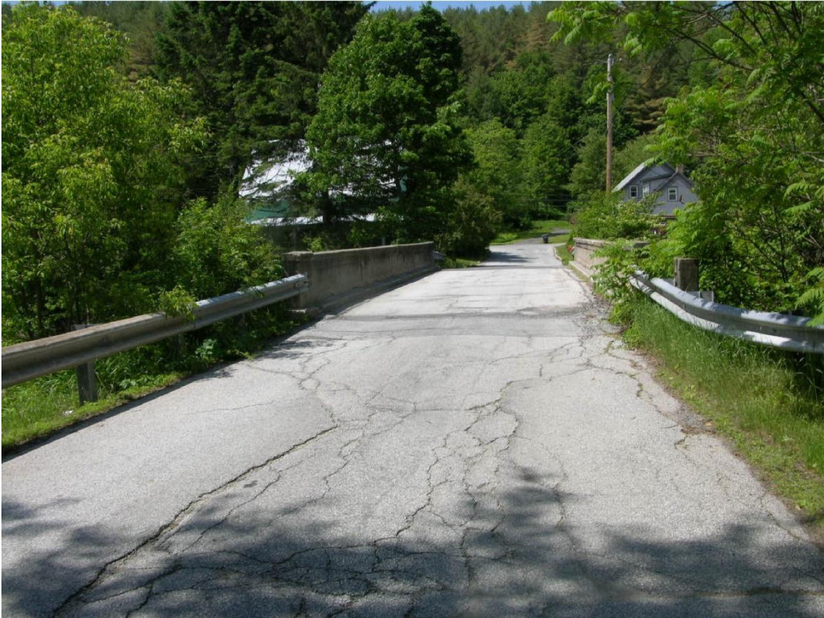
Looking west over the bridge at the patched joint
