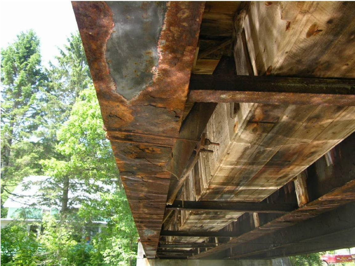
Girder Deterioration and Water Main Enclosure
