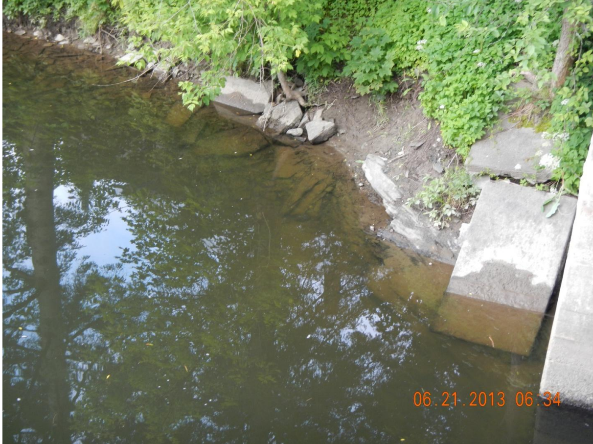
Figure 3. Potential bedrock outcrop and rip rap stone lining the eastern side of the bridge.
